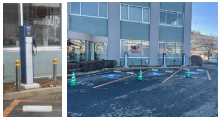
Electric vehicle chargers at an NAA Group company office
